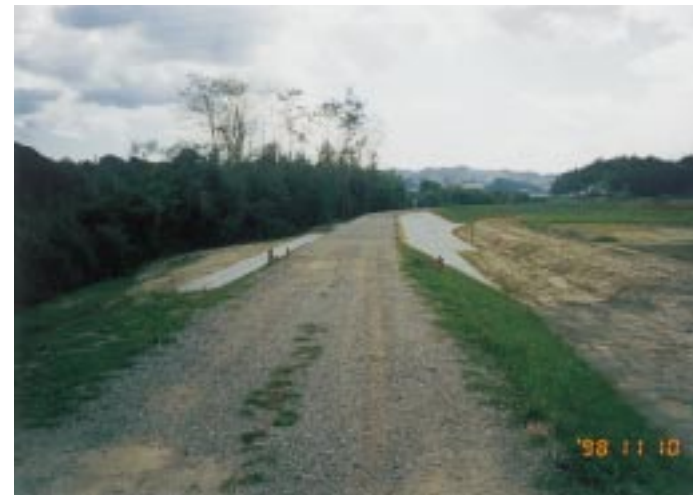
写真2 杉田川合流点破堤地点の復旧工事後の状況 Photo 2 Breaking point after the restoration works at the confluence of the Abukuma River with the Sugita River.
