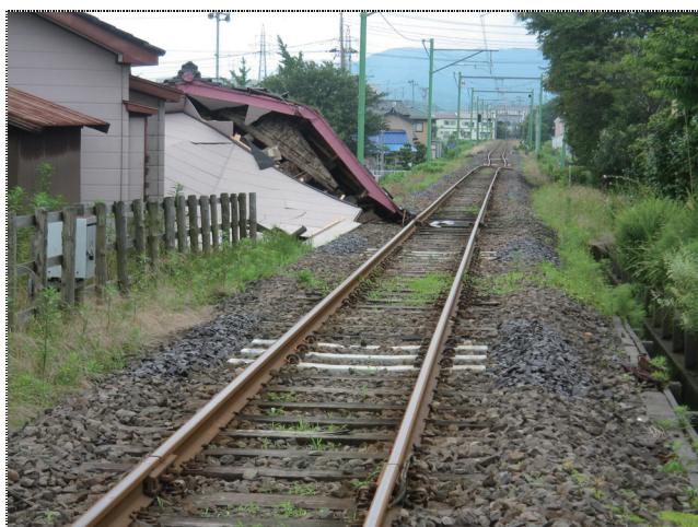
写真4 線路がうねった JR 越後線 Photo4 The railway was damaged by displacement of the ground (JR Echigo-line).
