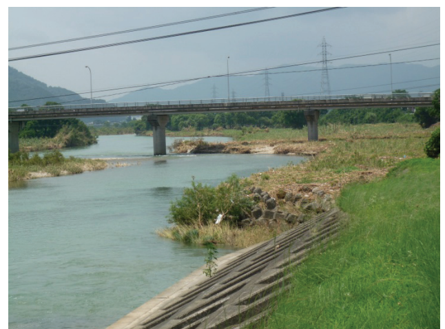
図 8 矢原河川公園付近の樫野川の洪水後の状況 Fig. 8 Condition of Fushino River after the flood near Yabara Riverside Park.
