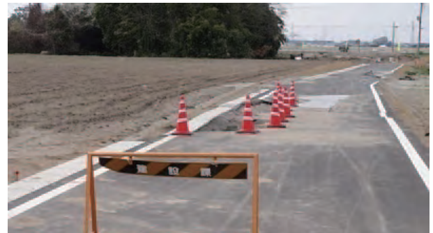
写真12 噴砂と陥没(常総市吉野) Photo 12 Sand boil and cave-in (Yoshino, Jyoso).
