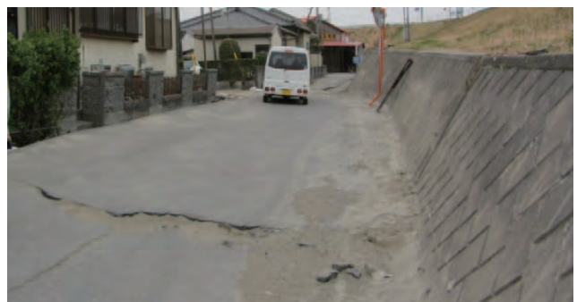
写真9 多量の噴砂による道路沈下(神崎町神崎本宿) Photo 9 Subsidence of a road by a large quantity of sand boil (Kozakihonsyuku, Kozaki).
