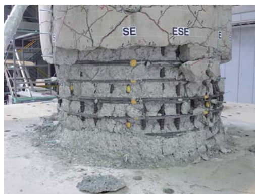
写真 61 C1-5(1)(2)(3)実験終了後南東面 Photo 61 Damage on SE face after C1-5(1)(2)(3) excitations.
