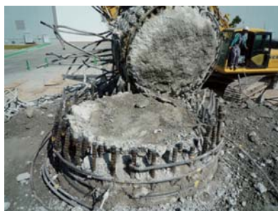
写真 8.1 破壊面 Photo 8.1 Failure surface after excitations.
