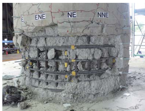
写真 63 C1-5(1)(2)(3)実験終了後北東面 Photo 63 Damage on NE face after C1-5(1)(2)(3) excitations.
