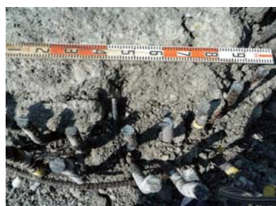
写真 8.2 帯鉄筋の定着部(SW 面) Photo 8.2 Bent hook of the ties after excitations (SW).
