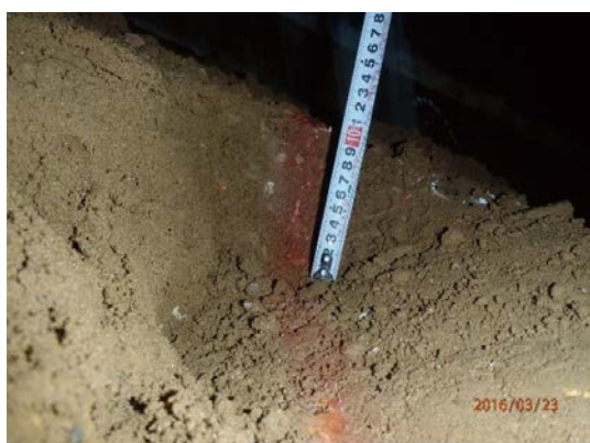
写真 22 前刃金上流法面クラック深さ測定状況 Photo 22 Measurement of the crack depth occurred in the upstream side in the case of sloping core zone.
