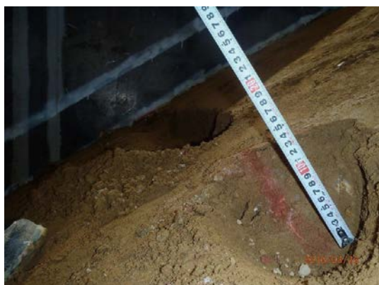
写真 24 前刃金下流法面クラック深さ測定状況 Photo 24 Measurement of the crack depth occurred in the downstream side in the case of sloping core zone.
